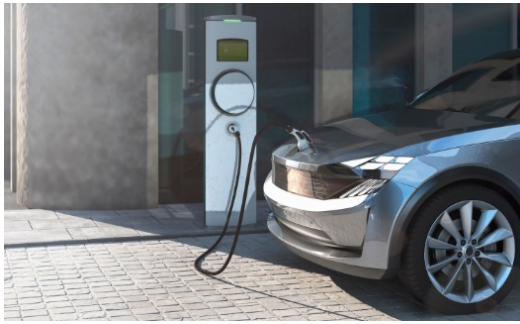
Figure 4 Infrastructure de chargement
